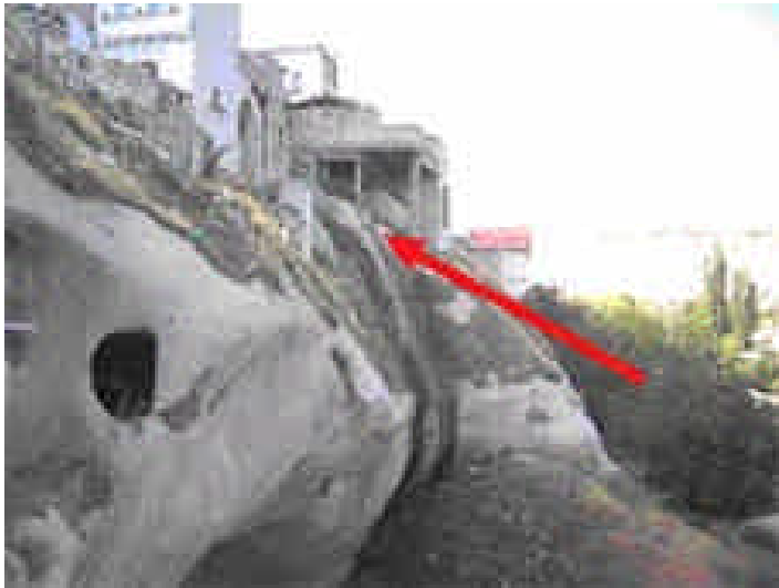
● Wastewater coming out of a tube falling in the valley
